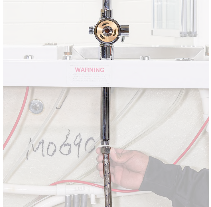
Tighten supply hose on the bottom of shower column
